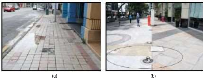
Fig.7 (a) and (b): Lack of maintenance of pedestrian walkway in JTAR (Source: Author, 2016)
