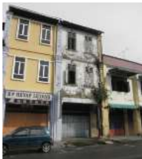
Figure 5: Shophouses in dilapidated state
